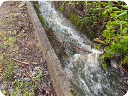
4 Disruption of natural water flow across the site. The past installation of culvert has disrupted the natural water flow and cannot withstand the volumes of water coming from the headland.
